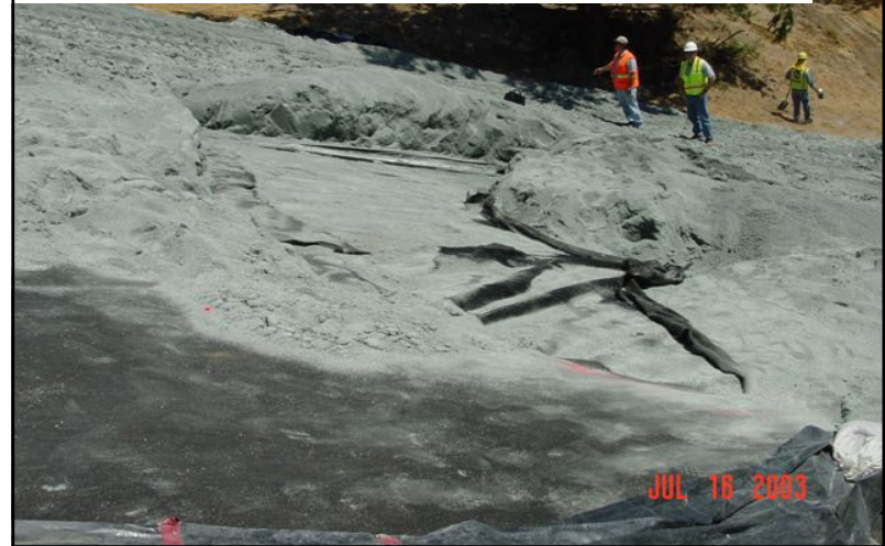
Landfill Cover Geocomposite Failure in California
