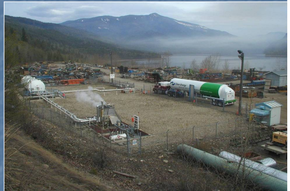
Terasen/Clean Energy – British Columbia
